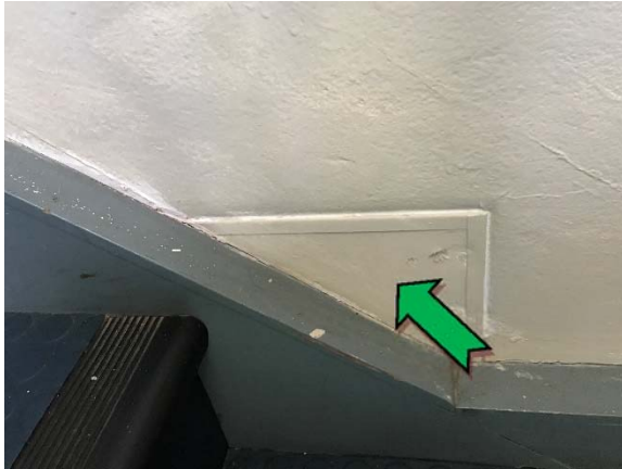
Photo 1. Interior, ground level, staircase, wall panels – non asbestos containing fibre cement sheeting.
