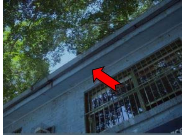
Photo 2. Exterior, north elevation, eaves – suspected asbestos-containing fibre cement sheeting.
